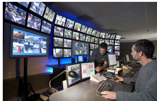
Figure 2. A control room for video surveillance (source [30])
